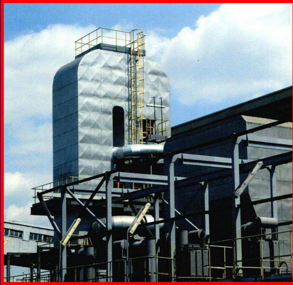
Operating Plant Rybnik, Poland
